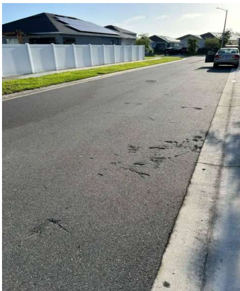
Road Damage on Cascade Drive
