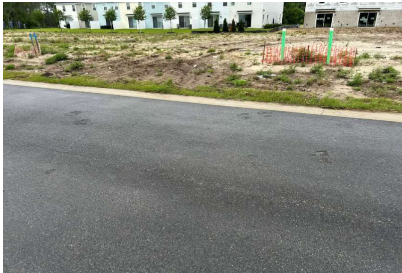
Asphalt Pitting on Sweet Sapling Court
