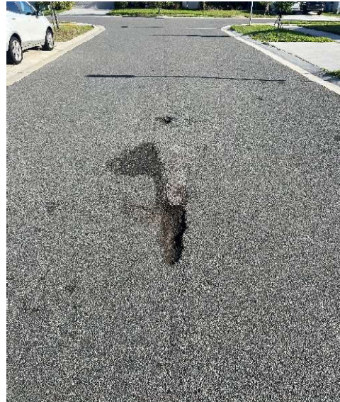
James Paul Rd. Pothole
