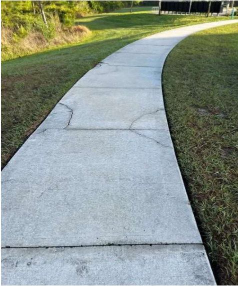
Cracked Sidewalk (Lily Lane, mail kiosk in background)
