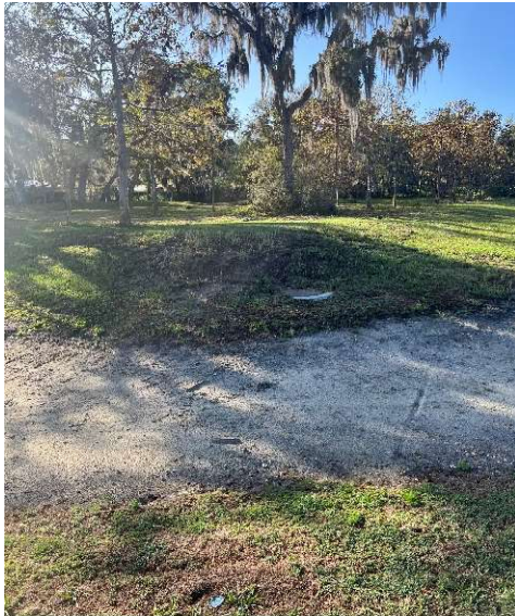
Pond 60 Soil Erosion
