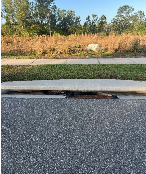
Sediment & Filter Fabric in Curb Inlet (typ.)
