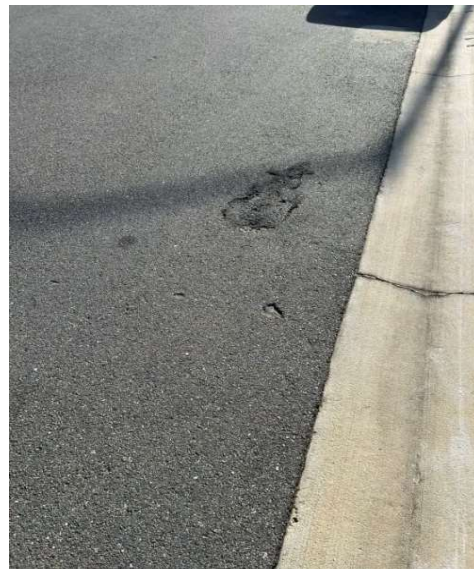
Road Damage on Orchid Drive
