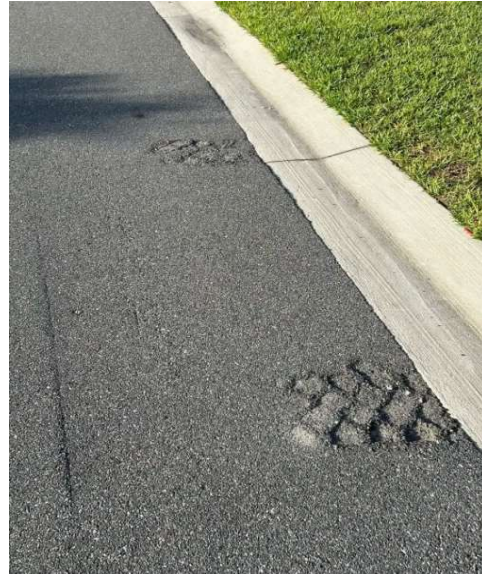
Road Damage on Oceania Avenue
