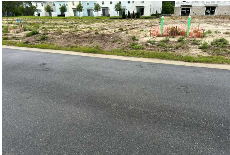
Asphalt Pitting on Sweet Sapling Court
