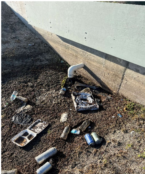
Pond 30 Clogged Orifice
