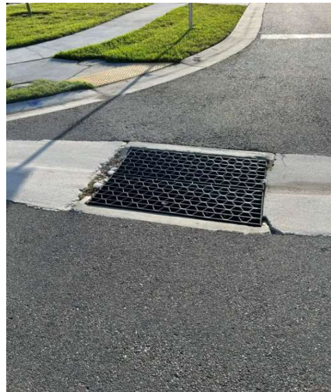
Damaged concrete at v-inlet (Brisbane Place and Cascade Drive)
