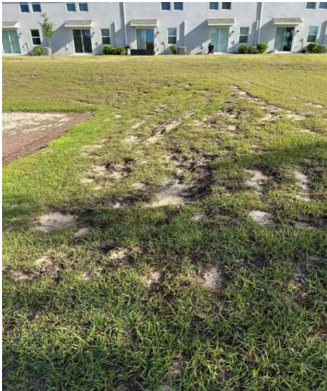
Pond 300 Eastern Bank Erosion
